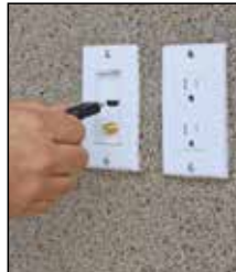
USB & Cable Hook-Ups Electrical Outlet
