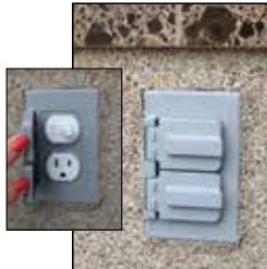
Light Switch & Extra Electrical Outlet
